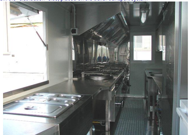
Interior view of the unit from the entry door: to the left, the cooking and distribution side to the right, the sink and fridges side
